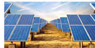
Figure 23: Spatial Setup of Large-scale PV system at Cochin Airport, India (source: sustainableinfacts.com )
